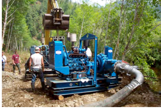
Photo 13 – Second pumping station
