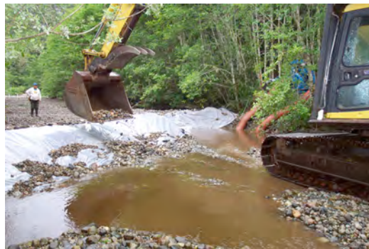
Photo 7 – Gravel plastic lined dam at first pumping station
